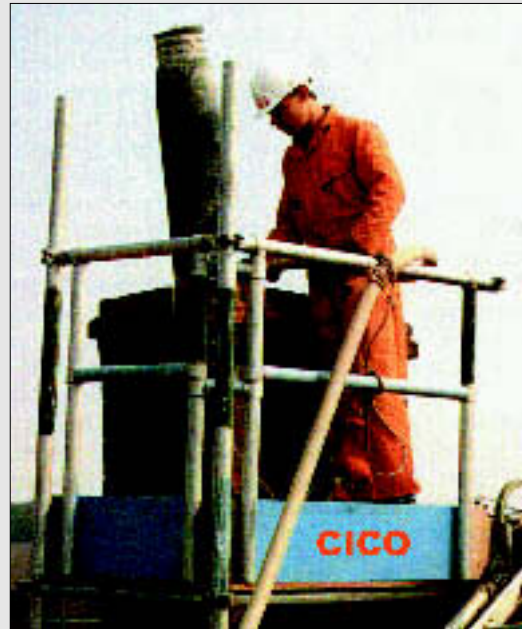
A CICO installer inspects work during the relining of an existing chimney
