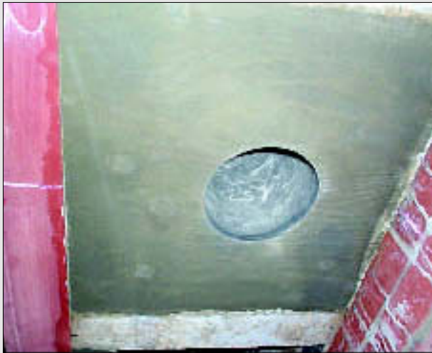
Lower end of a CICO cast-in-situ lining installed in a new property
